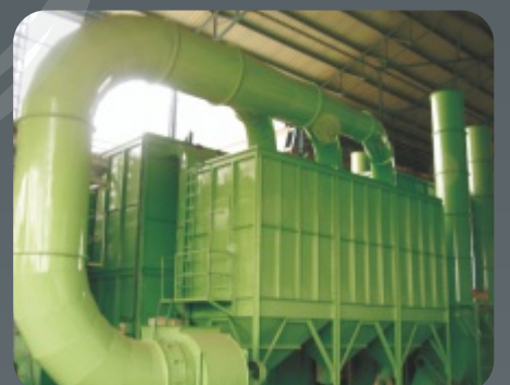
Fabric Bag Dust Collector at site for Blast Room
