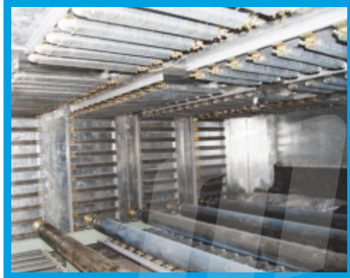
PRE HEATING CHAMBER
