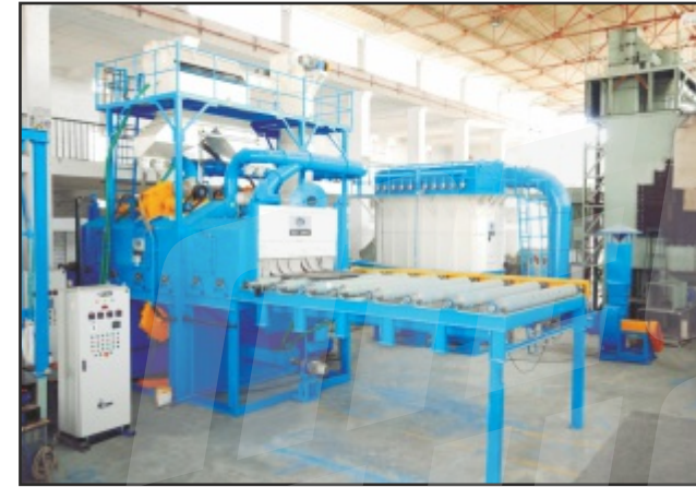
Tunnel Type 4 Wheel Shot Blasting M/c for Plate Cleaning
